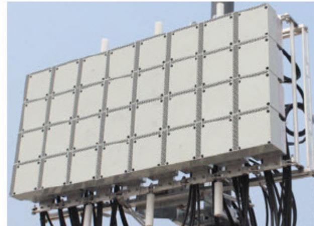
A massive MIMO antenna array for a Huawei 5G field trial.
