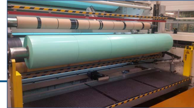
One of Mondi Gronau's plastic production machines, which deliver about 18 million tons of plastic and thin film products annually.
